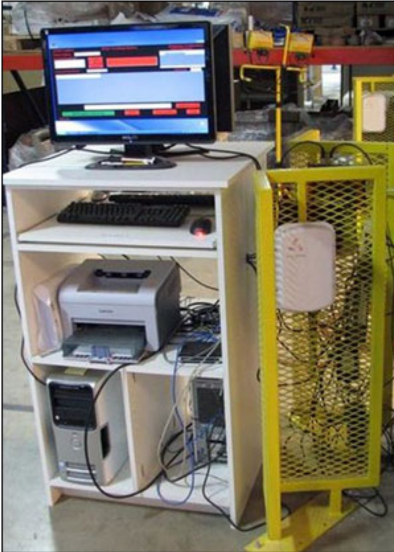
Each of Solid Comfort's RFID portals has an RFID reader and an antenna wired to a video monitor.
