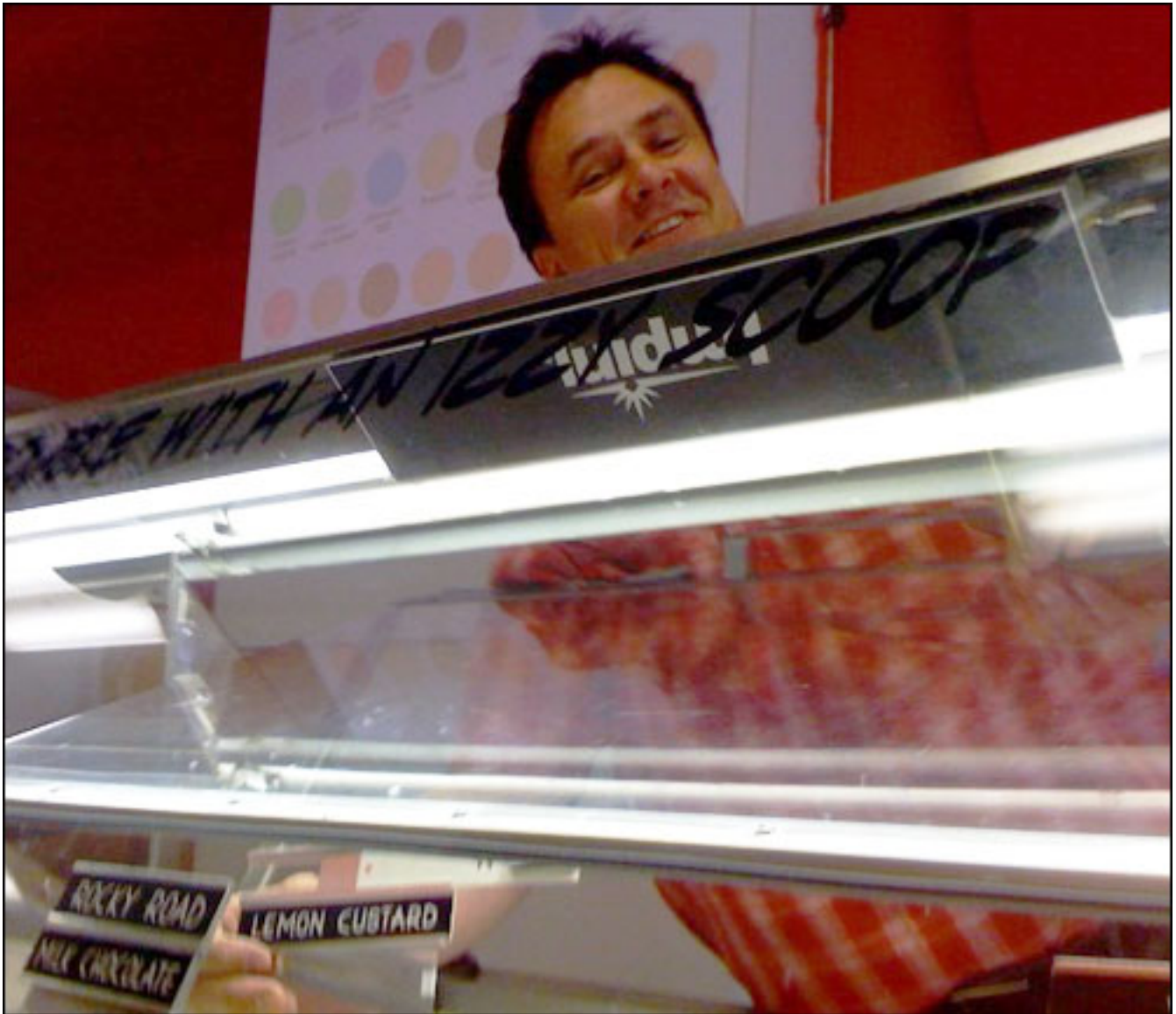
To read each flavor label's RFID tag, Izzy's installed Impinj reader antennas at the top inside of its display cases.
